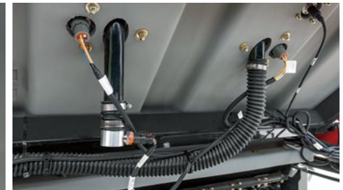
Tank pressure sensors.
